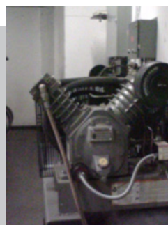
Air Compressor – Full Visible
