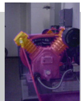
Air Compressor – AutoBlend™ Mode
